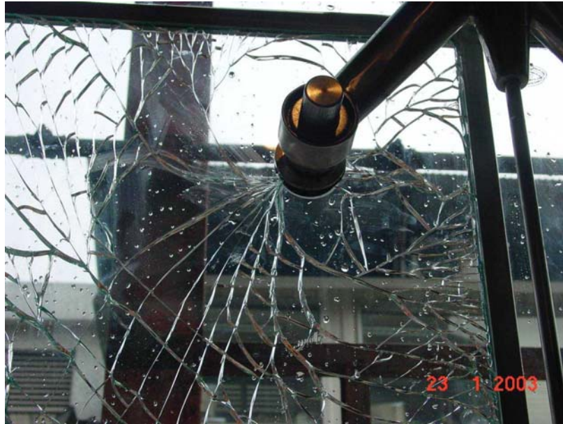
Figure 14: Glass failure during the performance test
